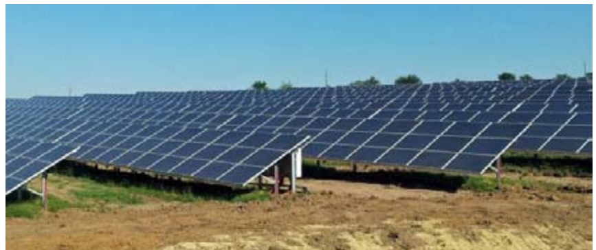
The Red Lands Roses Solar energy plant
