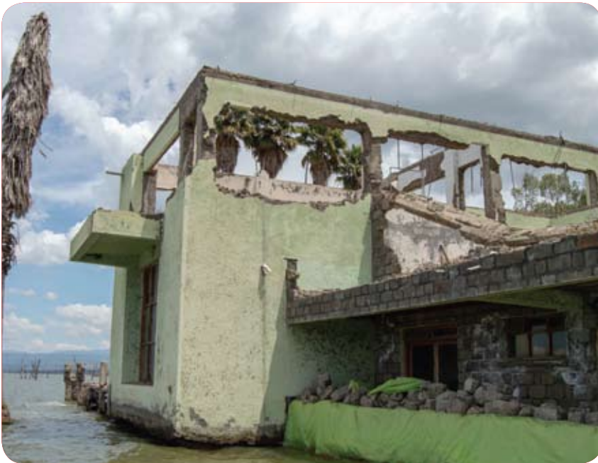
Illegal structure that was constructed in L. Naivasha
