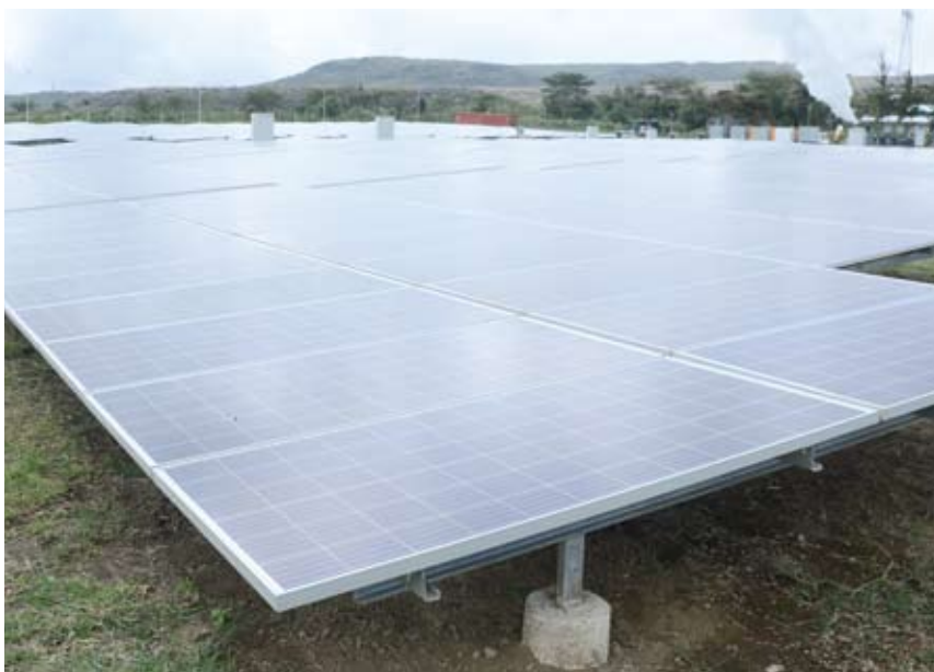
The 3000 solar panel launched by Oserian Development Company Limited with a capacity to generate 1MW
