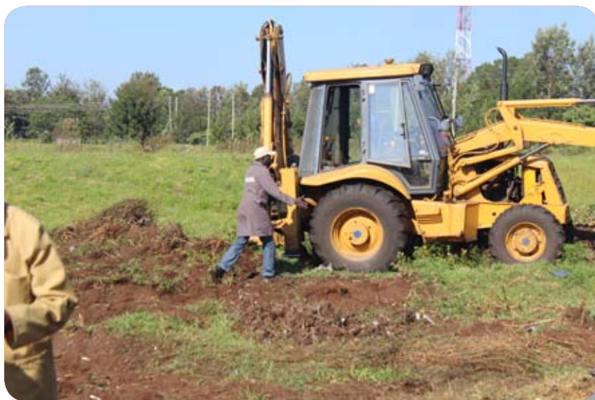
Leveling ongoing in one of the farms United Selections is putting up a solar powered system that will hold a capacity of 110 kilowatts
